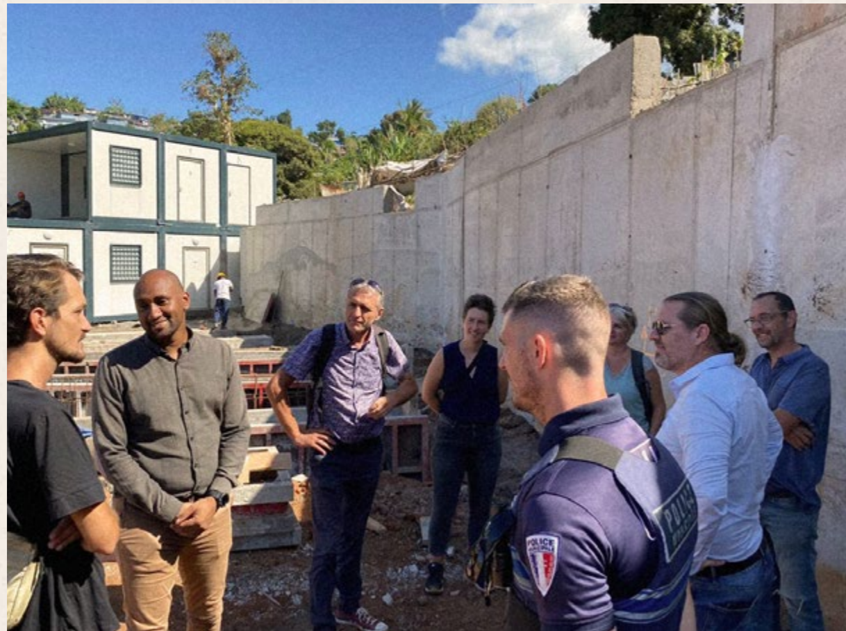
Stakeholder visit to construction site for temporary social housing, Majicavo Koropa, Mayotte, September, 2023. Photo: Anna Siegert
