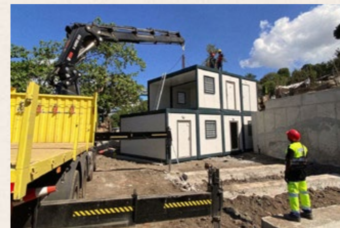
Construction of temporary social housing, Majicavo Koropa, Mayotte, September, 2023. Photo: Anna Siegert
