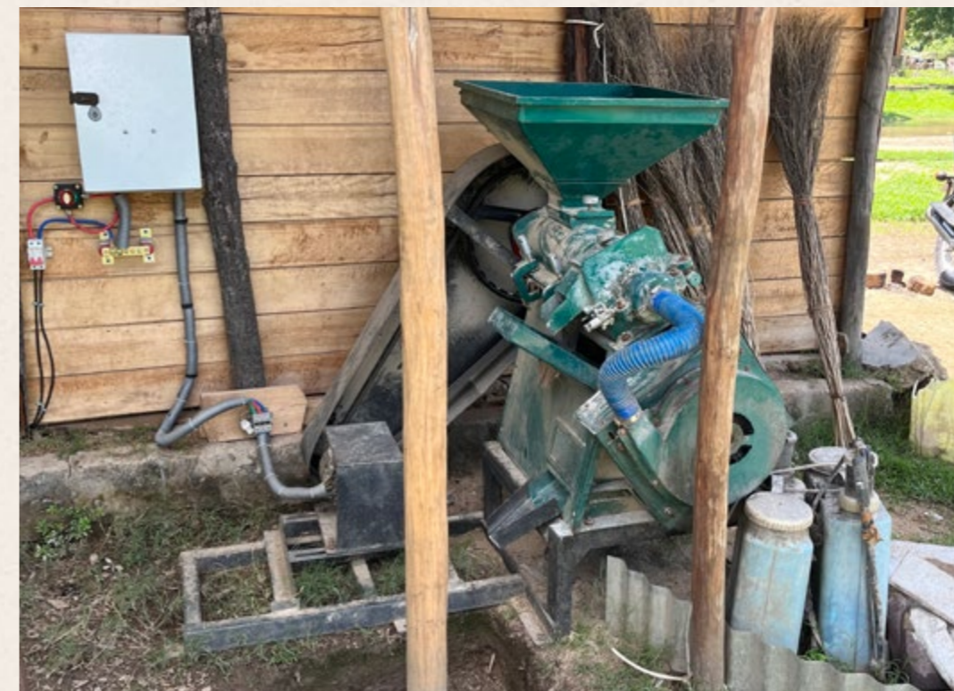
Solar-powered ICES with a rice huller enabling seasonal, community-based rice processing through a nanogrid. Antanananana, Madagascar, December, 2024, Photo: Philipp Baslik.
