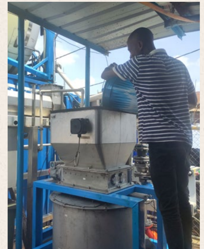
Waste manager, Abubakar, throwing organic waste into a grinder, to be fed into the bio-digester tank, which will turn the waste into biogas and liquid fertiliser, Freetown, Sierra Leone, May, 2024. Photo: Anne van Leeuwen.
